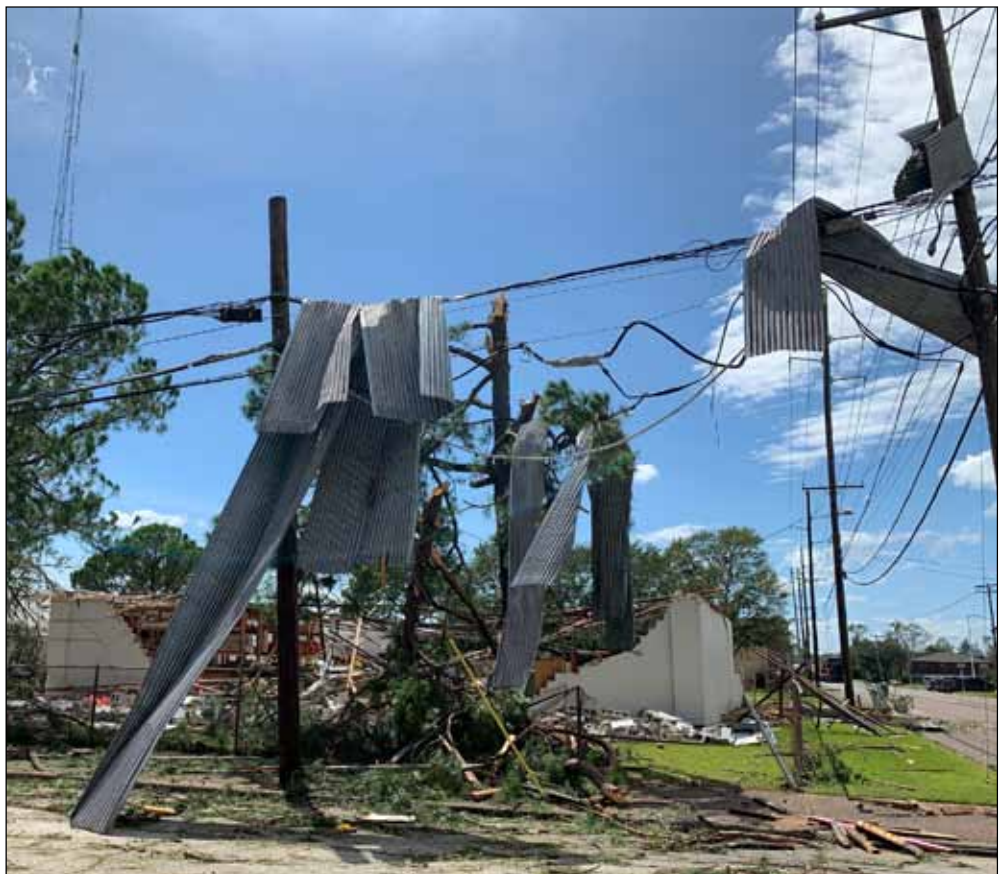
Metal from the roof of a destroyed Stark Foundation warehouse is draped over power lines at the corner of Front and 7th Streets Thursday afternoon. The building was a total wreck while a tall radio antenna behind it appeared unharmed by Hurricane Laura. RECORD PHOTO: Dave Rogers
