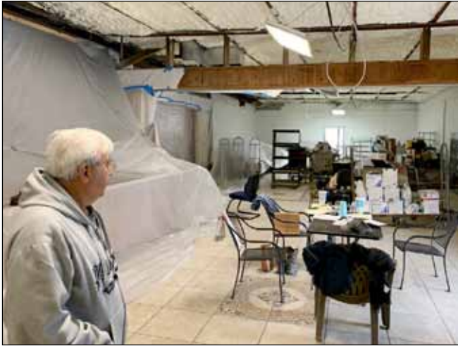
Robert Ramirez, owner of Robert's Meat Market and Steakhouse, 3720 W. Park Avenue in Orange, looks over the banquet rooms awaiting new ceilings and furniture after last summer's fire. RECORD PHOTO: Dave Rogers
